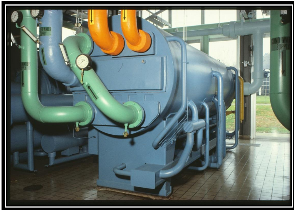
Figure 1. Absorption chiller providing chilled water in the Rueben Trane Building
